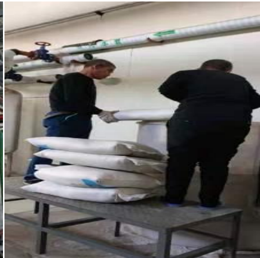
东区锅炉房软化罐加盐
